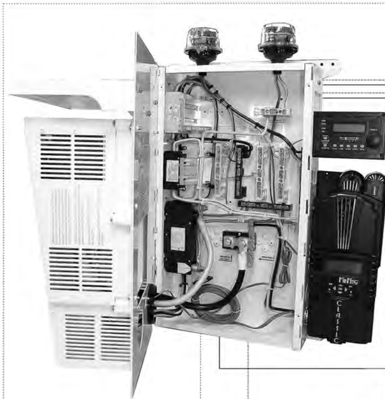
Interior View: MidNite Solar Disconnect with Magnum MS4024PAE mounted on door.
